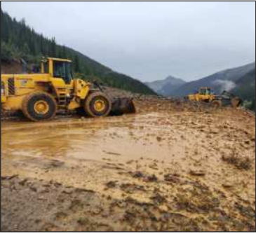
photo by CDOT Mudslide on Red Mountain pass last week
